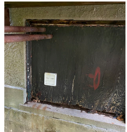
Photo 3. Plywood panel needing air sealing
