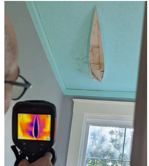
Photo 1. Signs of possible roof leak
