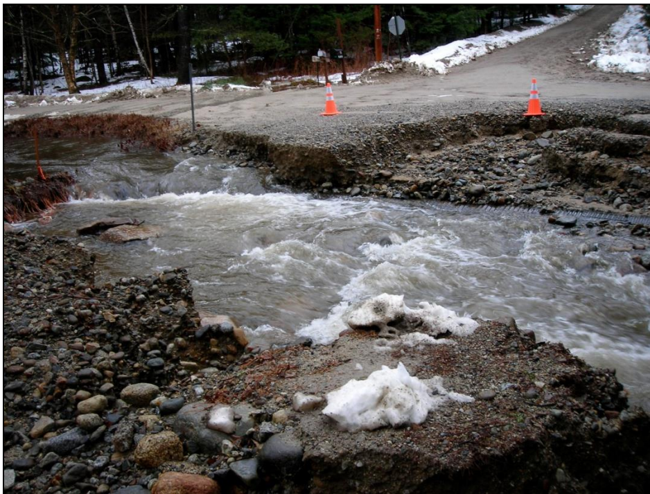
West Joppa Road and Parade Ground Cemetery Road Culvert Overflow
