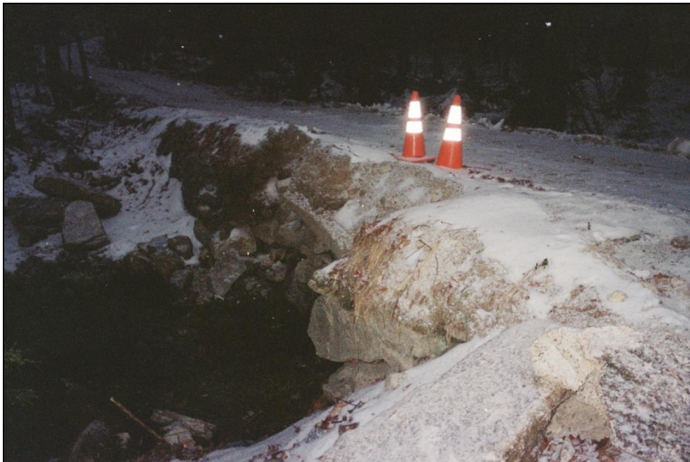
Unidentified Road and Culvert Icy Conditions, December 2008
