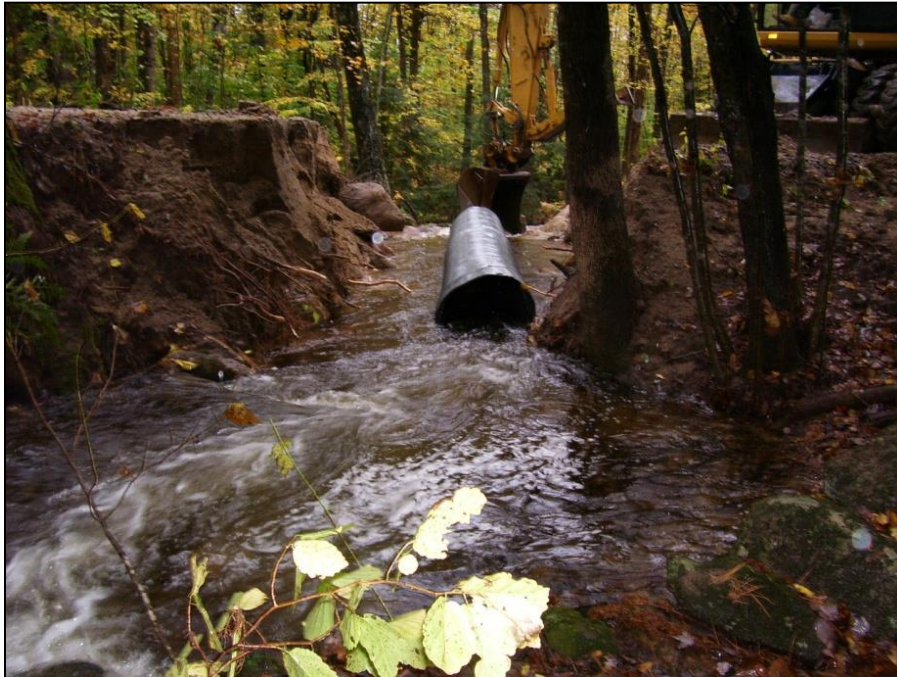
Culvert Washout on Ladd Lane
