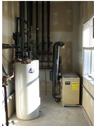
Bradford hot water tank uses preheated water from boiler and appears adequate.
