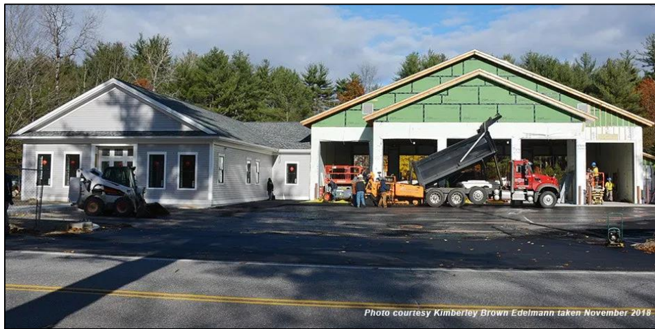
Warner Fire and Rescue Building Under Construction Nov 2018 at 148 West Main Street (Photo by Kimberley Brown Edelmann, accessed online 02-19)
